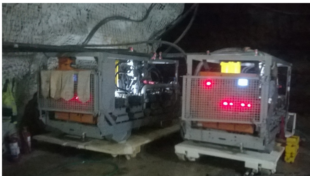
The pumps at the drill site
