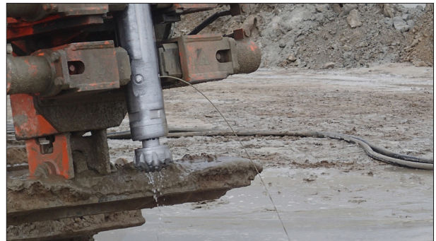
The jet grouting hammer after completing one column. Some grout is still seeping from the monitor.
