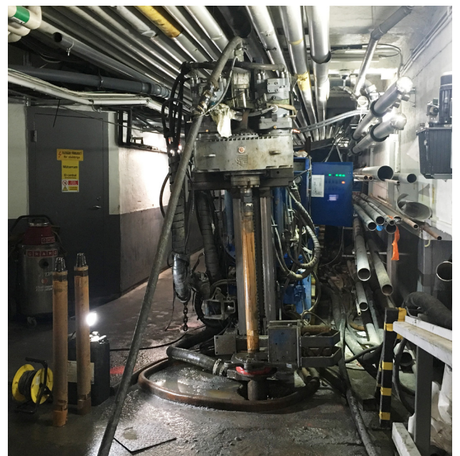
Wessman Drilling Solutions drilling in the basement of the building at Stureplan
