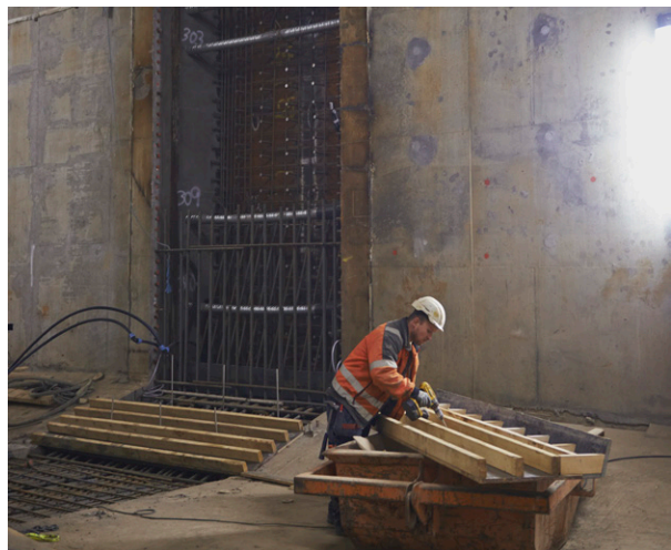
The joint between tunnel element 2 and 3 before being filled with concrete. The horizontal cable packages are clearly visible.
