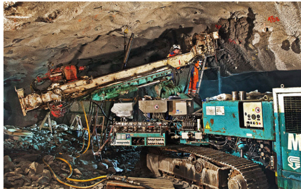
Aligning the drill rig for the next rock anchoring hole (Photo by Hans Ekestang)
